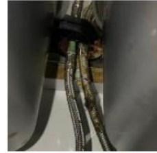
Calcification noted to fitting and rust noted to braiding.
