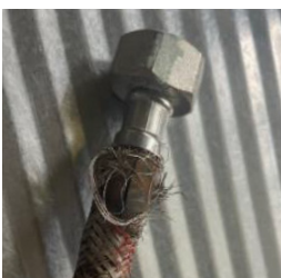
Example of failed flexi-hose due to rust and corrosion.
