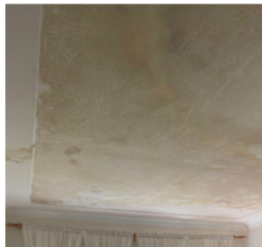
Water damage to ceilings, walls and contents
