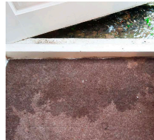
Water-logged carpet and underlay which may be unrestorable
