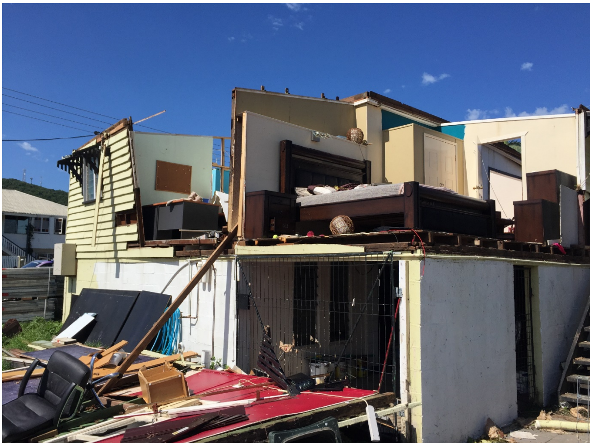
Figure 1. Severe roofing damage from Cyclone Marcia in 2015 due to inadequate load capacity at the rafter to top-plate connection
