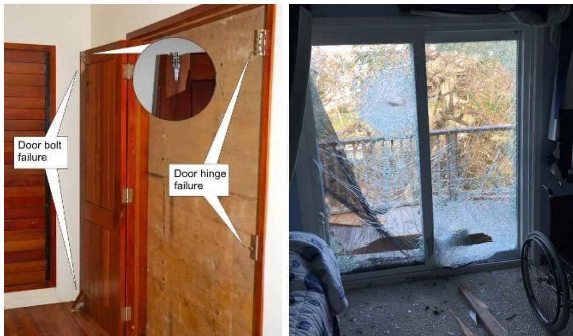
Figure 2. Door bolt and hinge failure from Cyclone Yasi in 2011 (left) and wind-borne debris failure of impact-resistant glass door from a tornado during Hurricane Irma in 2017 (right)
